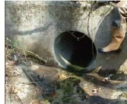
The drainage to this outfall most likely has a high nutrient concentration. The cause may be an illicit discharge, but may be excessive use of lawn chemicals.
