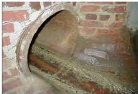
Bacterial growth at this outfall indicates nutrient enrichment and a likely sewage source.
