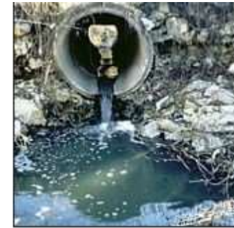
High severity suds Rating: 3 Sewage
